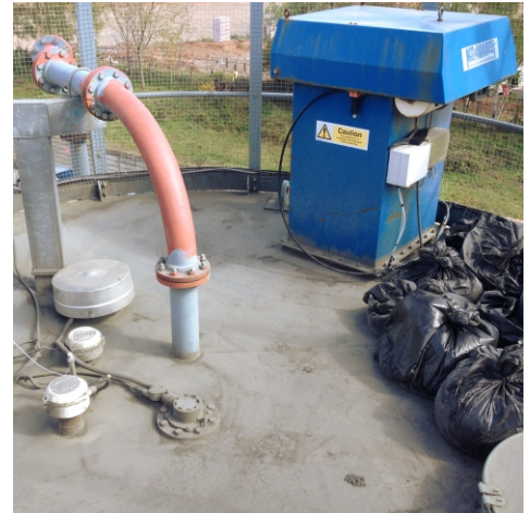
Despite correct safety equipment cement was still being deposited on top of this silo. Seven bags of product were removed prior to this photo.
