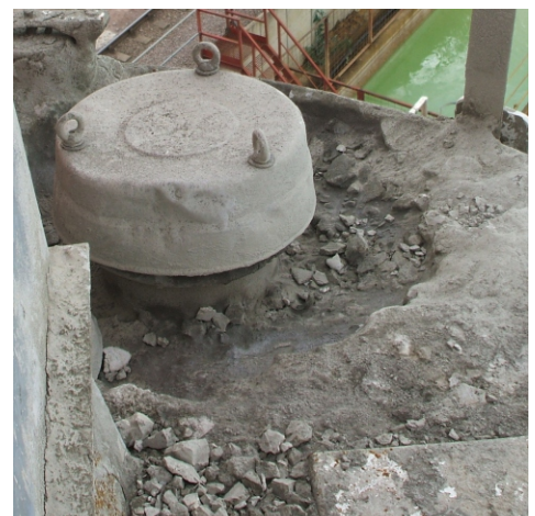
This PRV has been replaced twice in 12 months, but the cement visible is due to a faulty filter. This was missed by incompetent service engineers.
